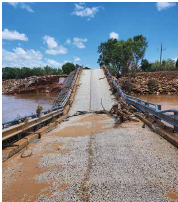
Forming an integral part of WA's Great Northern Highway, the Fitzroy River bridge collapsed and will take years to repair effectively splitting the Kimberley in two.
